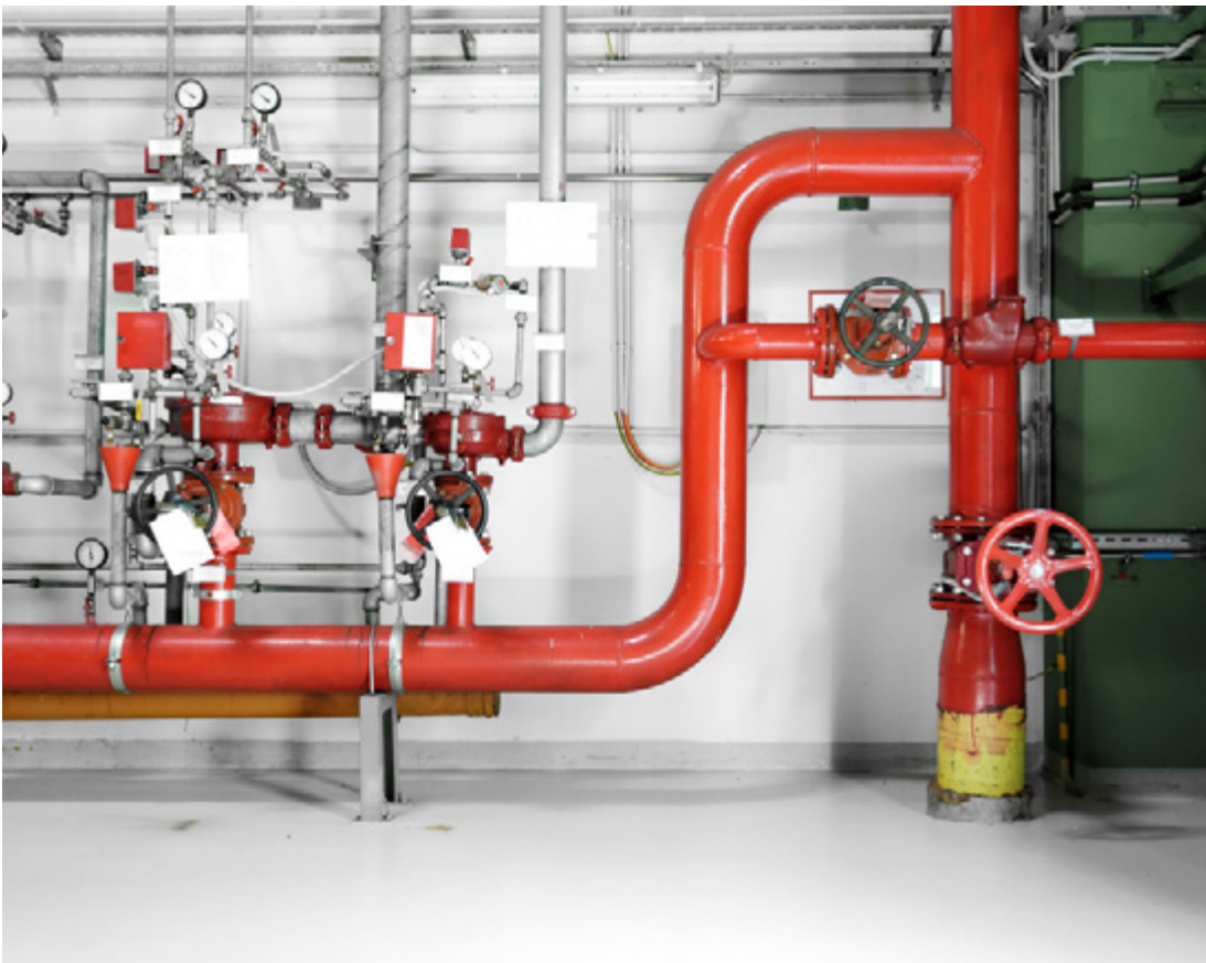
Industrial fire protection systems were developed, in part, due to early risk management efforts related to fires and explosions.
